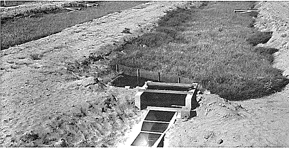
Effluent channel in Salt River bed west of Phoenix, carrying a flow of about 50 mgd (about 80 cfs).
